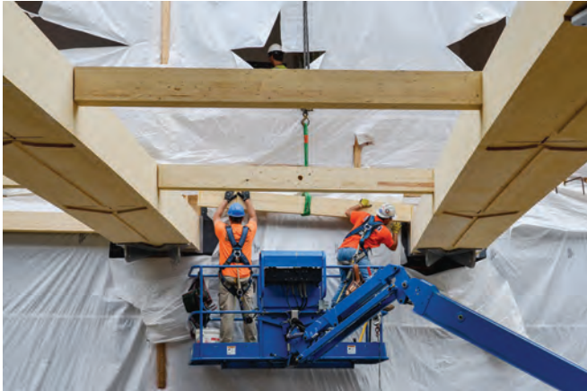
FIGURE 5-43: Setting beams at the John W. Olver Design Building, UMass Amherst Image: Alex Schreyer
