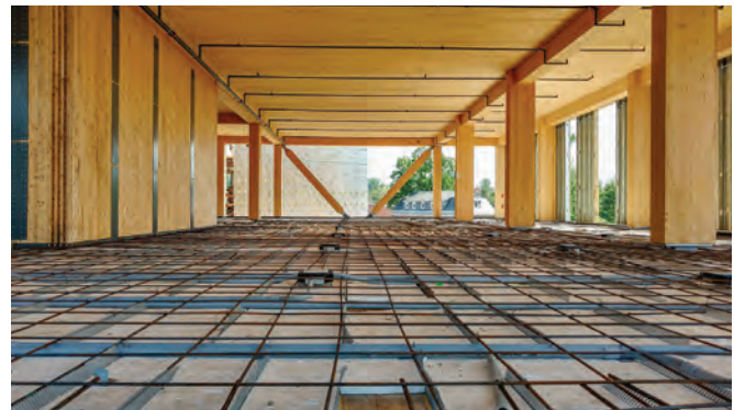
FIGURE 5-47: (Top) Panels with pre-installed shear connectors being installed and subsequent shoring on the TCC system.
