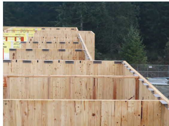
FIGURE 5-11: Wide angle view of CLT shear wall brackets installed prior to floor deck placement
