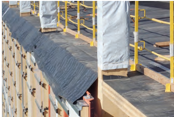
FIGURE 4-5: Vapor-permeable water-resistant barrier on CLT floor panels, draped over the wall system below to deflect water from the lower floors
