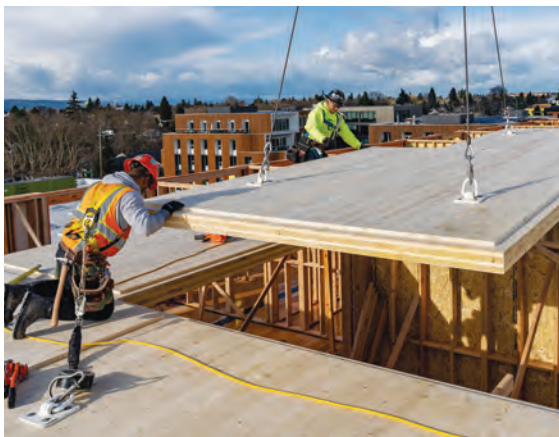
FIGURE 5-44: Setting floor panels at The Canyons in Portland, OR Image: Kaiser+Path, photo Marcus Kauffman, Oregon Dept. of Forestry
