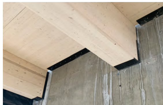
FIGURE 5-32: Note the gap between the mass timber and concrete Image: Ricky McLain, WoodWorks
