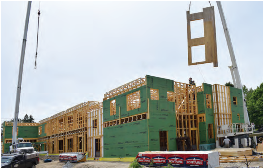
FIGURE 5-26: CLT elevator shaft walls flying into place in light-frame hybrid Image: Avesta Housing
