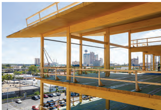
FIGURE 5-5 Guardrails installed at The Soto Image: Cheyne Smith, BOKA Powell
