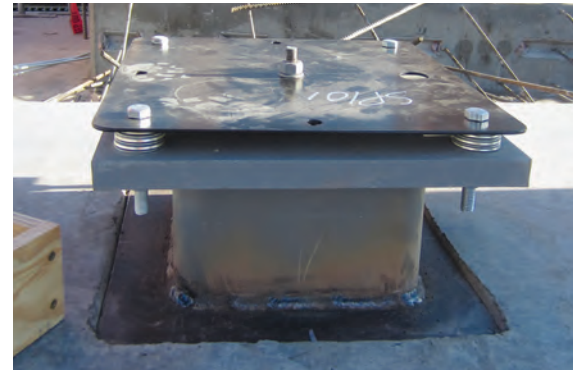
FIGURE 3-5: Column base connection with vertical adjustability. The column has a recessed base and hides the connection from view.
