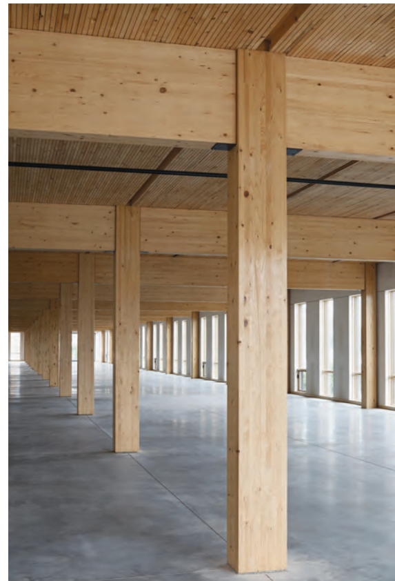
FIGURE 5-23: Column-to-column connection at 111 East Grand in Des Moines, IA Images: Neuman Monson Architects; photo Mike Sinclair
