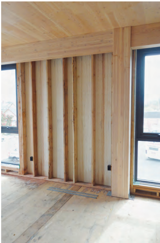
FIGURE 5-24: CLT and glulam construction with fire retardant-treated light-frame infill walls at Carbon12
