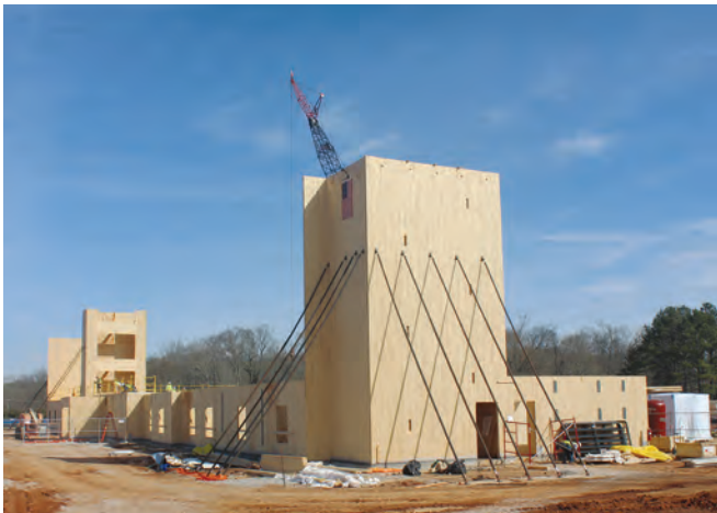
FIGURE 5-46: Three and a half-story stair shaft walls required engineer approval of temporary bracing and additional foundations outside the building footprint.
