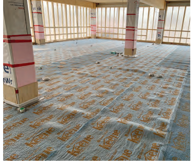
FIGURE 5-52: Column protection and acoustic membrane before concrete topping is poured Image: Anthony Harvey, WoodWorks
