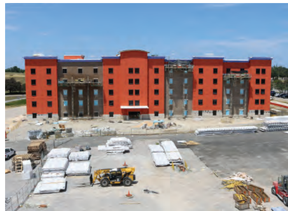
FIGURE 4-3: Staging area; CLT exterior wall façade with field-applied self-adhered water-resistive vapor permeable air barrier Image: Jeff Morrow
